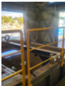
① Fall-Prevention Safety Fence
