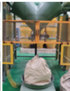
① Safety Fence for Rotating Machinery
